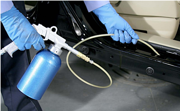
A typical recommendation for treating the backside of a repair is applying anti-corrosion compound with a wand through existing holes.
