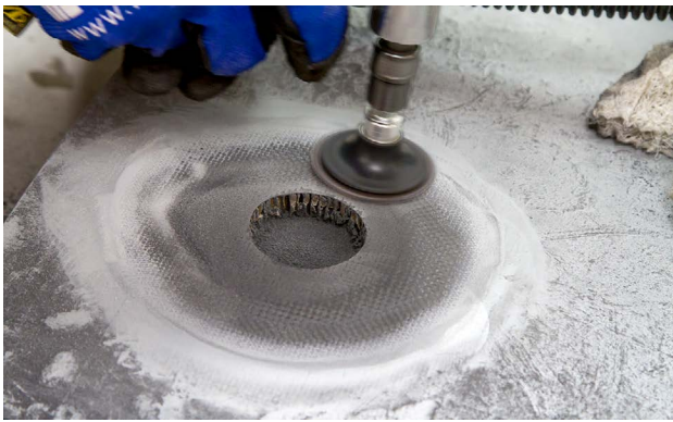
After the filler is removed, the repair taper can then be created.
