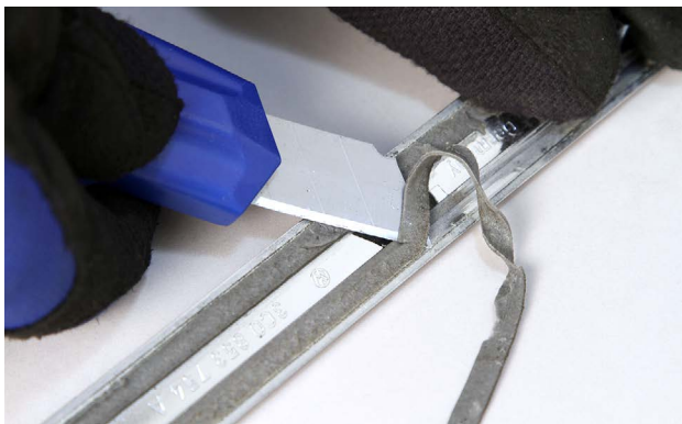
The adhesive is being removed from the molding using a razor blade.
