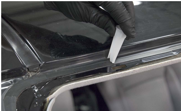
The technician is holding the pre-cut nozzle up to pinchweld wall to see if the triangle peaks just over the roof line.
