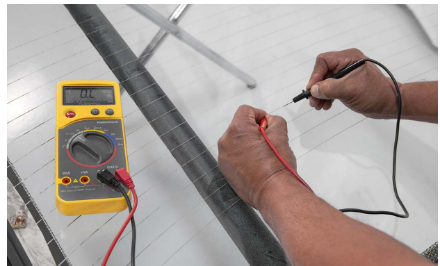
A continuity test shows "out of limits" confirming that there is a break in the grid line.
