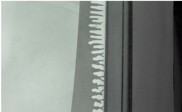
This is a delamination problem within the glass and cannot be repaired.
