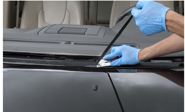
Pulling on the urethane during final trim helps assure the existing urethane is bonding well.
