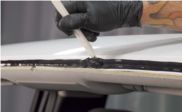
Paddling the urethane seals the start and stop points to prevent leaks.
