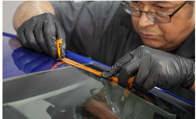
The technician is applying tape on the windshield at the roof line to help line up the glass when the urethane is on the pinchweld.
