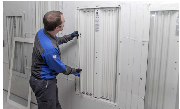
Spraybooth light bulbs should be replaced on a regular basis.
