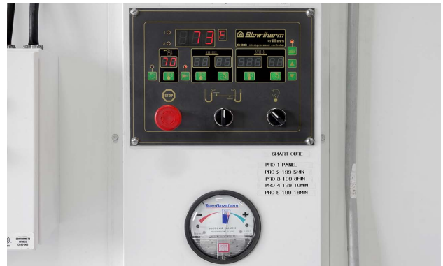
Spraybooth temperature can be adjusted to match refinish material requirements.
