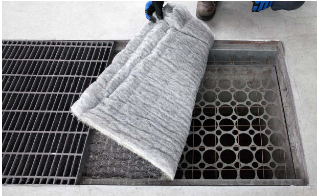
Spraybooth filters should be replaced on a regular schedule.
