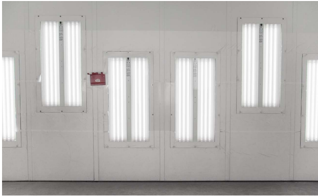
Spraybooth lighting should be as close to natural daylight as possible.
