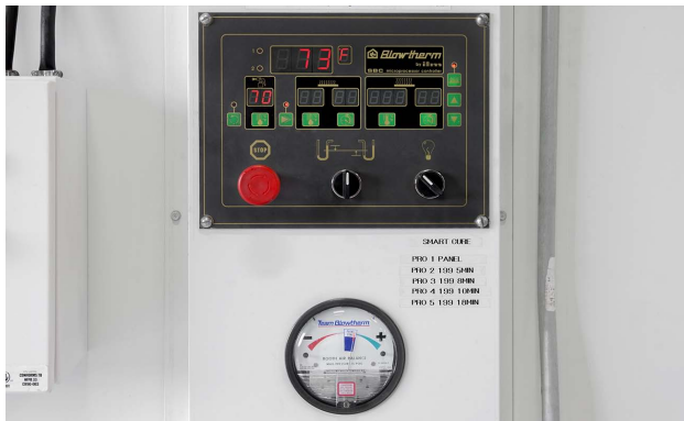
The internal spraybooth temperature can be adjusted at the control panel.
