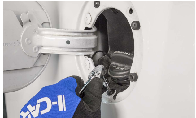
The fuel filler neck is being disconnected for box removal on this truck.
