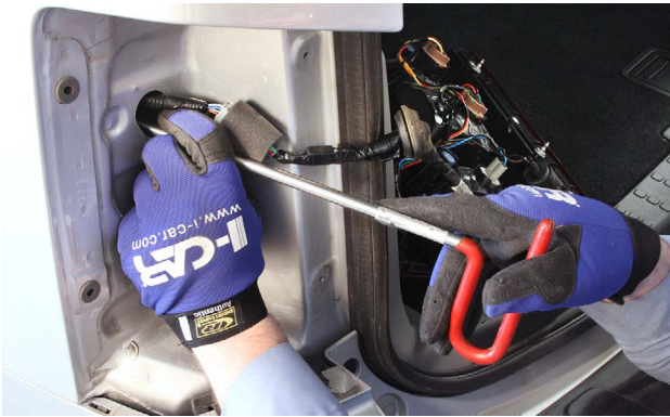
The tail lamp mounting area is a common location used to access the backside of the quarter panel.
