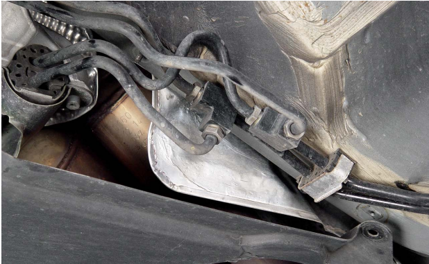
These fluid lines and distribution blocks for the hydraulic height control system are located where they are susceptible to damage in a collision.
