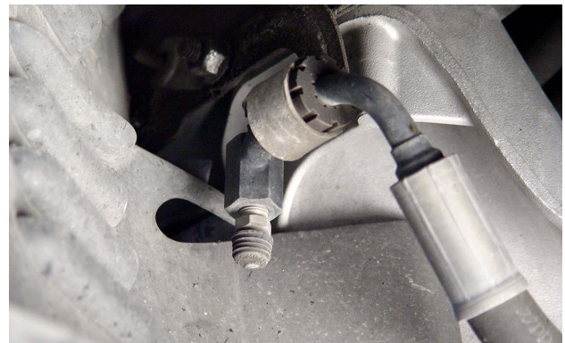
The bleeder valve for this hydraulic fluid line has a protective rubber cap.
