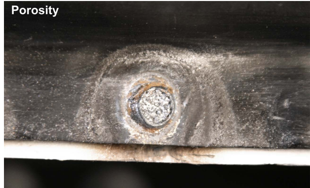
Welds with porosity are indications of a weak weld joint.
