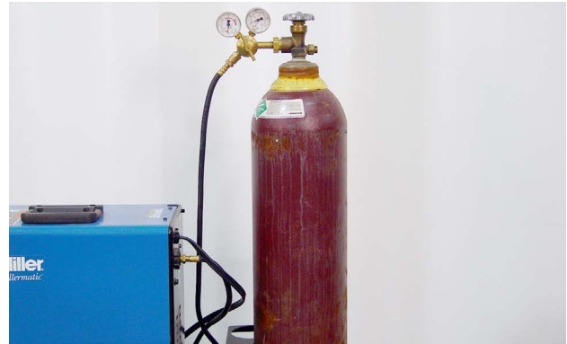
The shielding gas is stored separately from the welding machine in an external cylinder.
