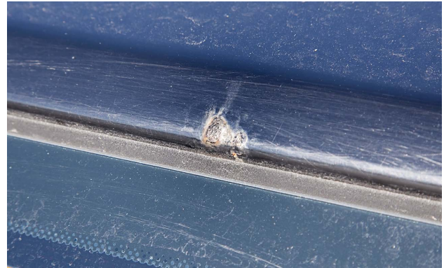
This mild corrosion issue must be repaired before a refinish is applied.
