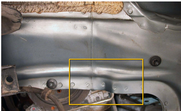
This rail shows a bend in the lower flange area.
